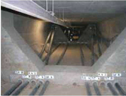
HDPE ducts for external prestressing
