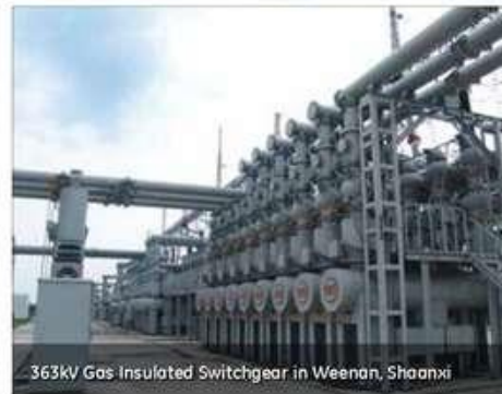
363kV Gas Insulated Switchgear
