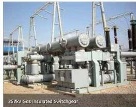
252kV Gas Insulated Switchgear
