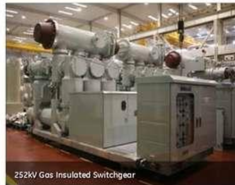
252kV Gas Insulated Switchgear
