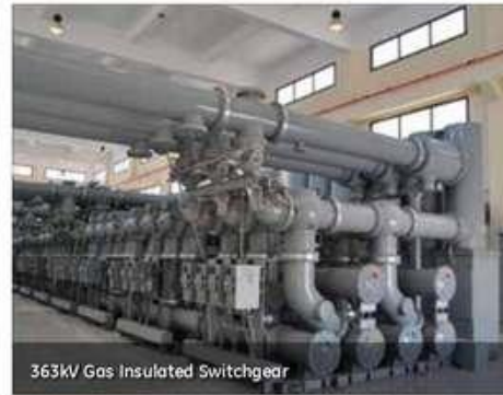
363kV Gas Insulated Switchgear at Golmud Substation
