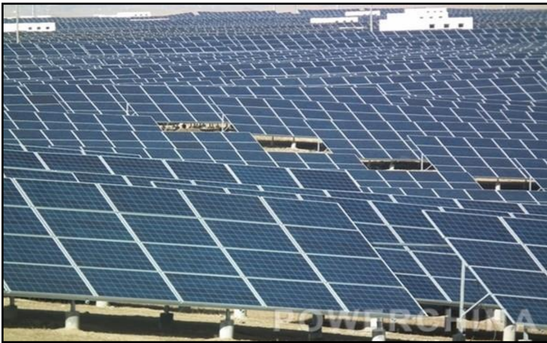
Figura 12: Longyangxia Hydro – Solar PV Station. 850 MW. China.
