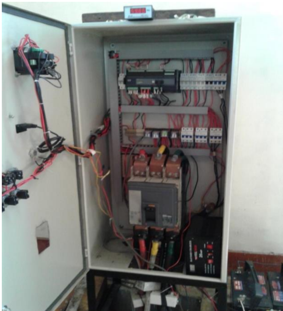
Figura 6: Tablero de control Central Lurini
